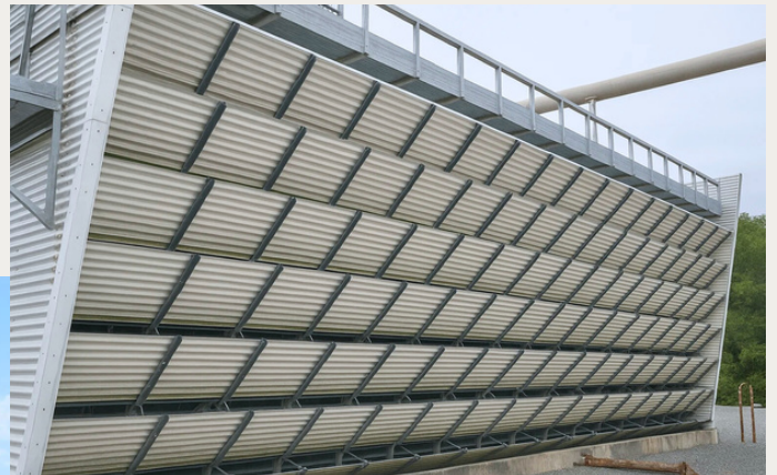
HVAC Ventilation Grilles
