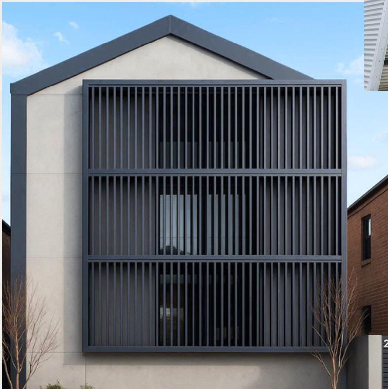
Air Conditioning Louvers
